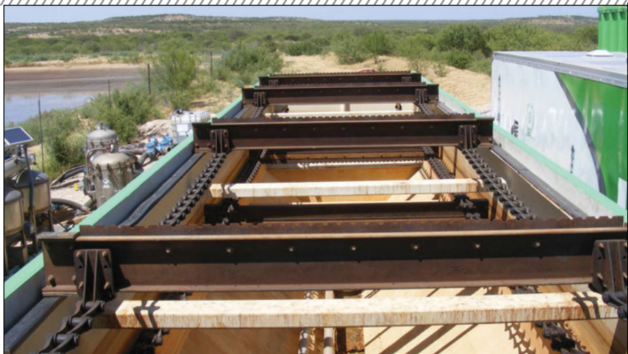
Scrapers remove solids on top of the unit where bubbles are formed.
