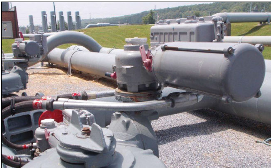
□ Electric actuators at a Williams natural gas pipeline facility
