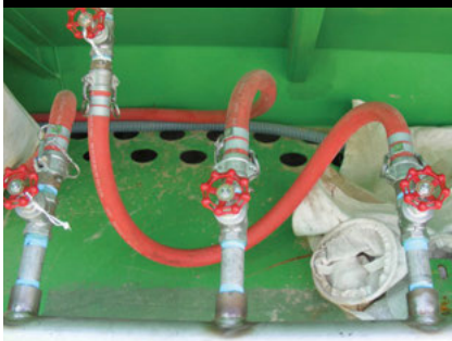
A gate valve introduces air to the DAF unit.
