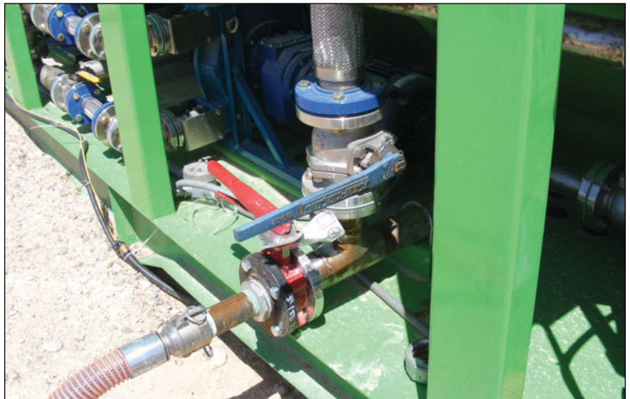
□ A butterfly valve (red handle) and a ball valve (blue valve) on the sump pump take waste out of the frack water
