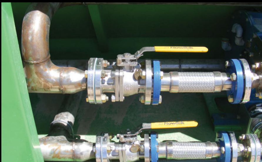
□ Ball valves connect to air floatation that goes to the DAF unit.
