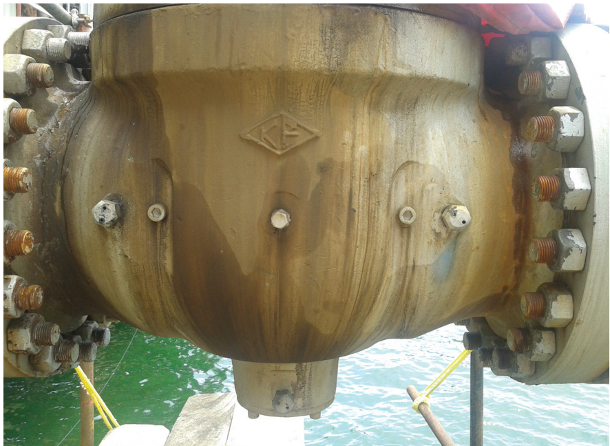
□ This top-entry ball valve has a bonnet leak.
