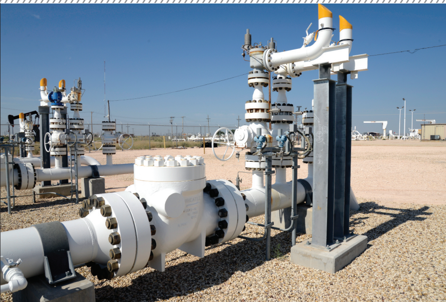
□ This is the termination point for the incoming pipeline from New Mexico that brings CO 2 to the field at a pressure of around 3,000 psi. The check valve and redundant pressure relief valves are critical for protecting the piping system from backflow and overpressure.
