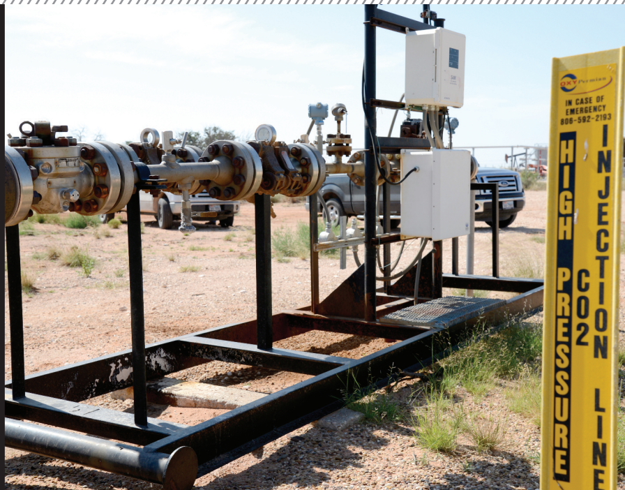
□ A typical Permian Basin injection manifold found just upstream of the wellhead is where incoming, very-high-pressure CO 2 and water are alternately fed into the Christmas tree and down into the oil-bearing formation.
