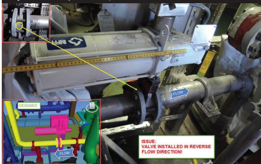
□ Figure 3. Actuated butterfly valve installation problem
