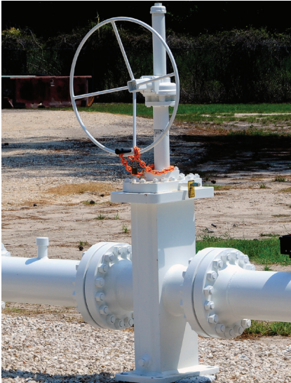
□ API 6D pipeline valves are addressed in one of the new IOGP standards addendums.
