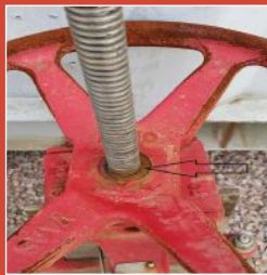
Corrosion of stem nut may increase operating torque
