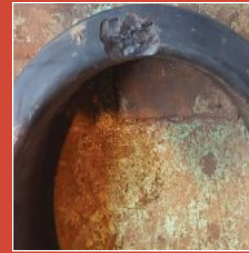
Push-through seal valve seat damaged in face area by elastomer deterioration
