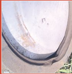
Erosive wear on valve body caused by abrasive slurry
