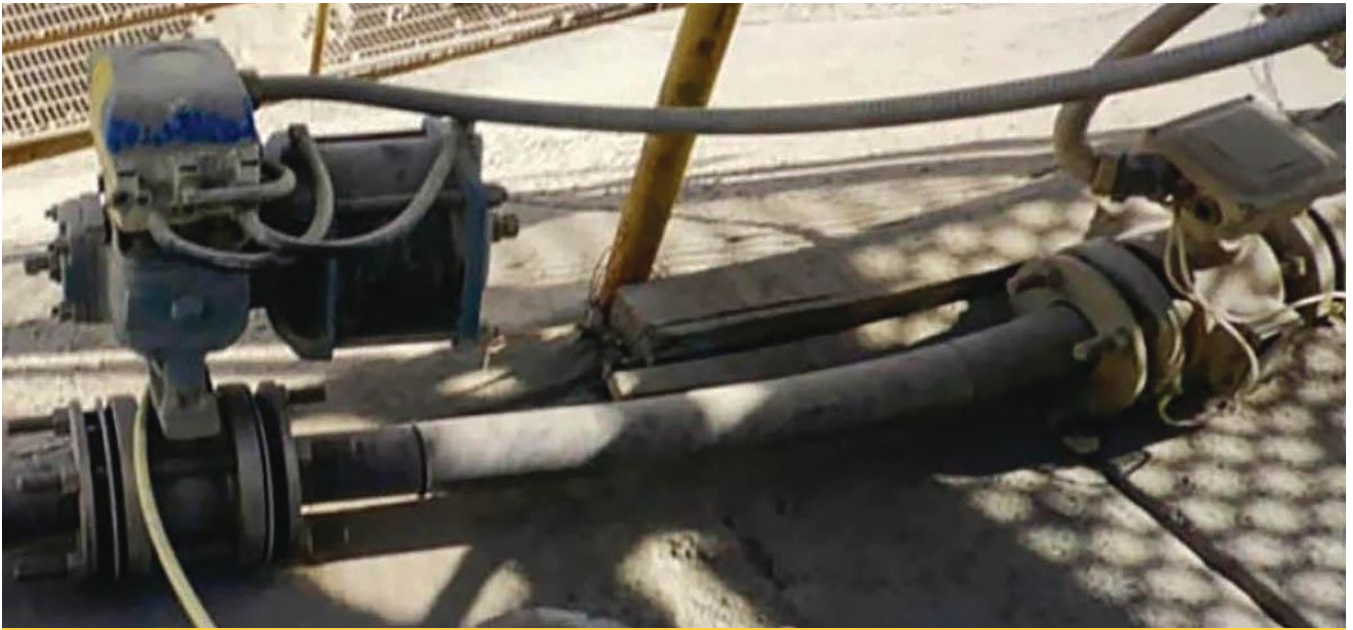
Figure 3. A copper mine installed a 2-inch rotary control valve body in its acid raffinate control on heap leach pads. When the mine was ready to increase flow capacity, it changed the valve seat trim size thereby eliminating labor-intensive and expensive piping changes.
