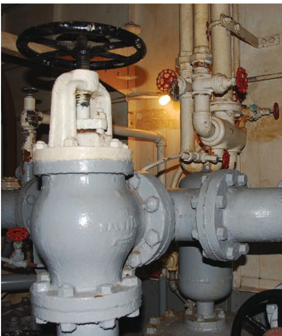
Figure 3: An angle globe valve in a marine application
