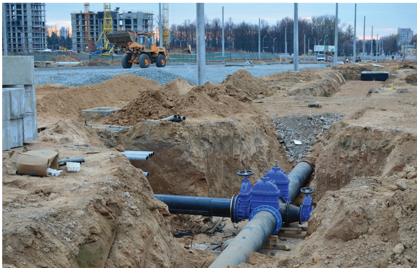
A municipal water system under construction – a sight in many cities and towns with the influx of government funding.
