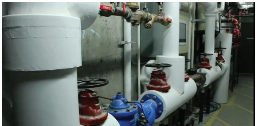
Sewage heat recovery system valves
