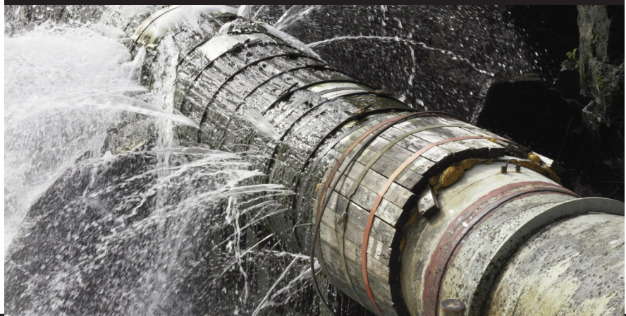
□ The nation's water infrastructure is in need of immediate help. Smaller electric actuators allow responsive centralized control to manage pressure in the distribution pipework for leakage mitigation.
