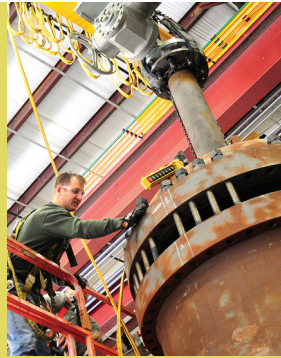
Large valve repair takes the right mixture of skill and materials handling capabilities. This 48-inch pipeline gate valve under assembly weighs in at just under 20 tons.
