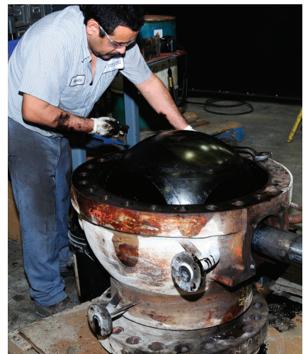
Specialty valves, such as this metal-seated coker ball valve are very expensive so end-users and owners of these high-ticket items have them repaired as many times as possible before replacement.
