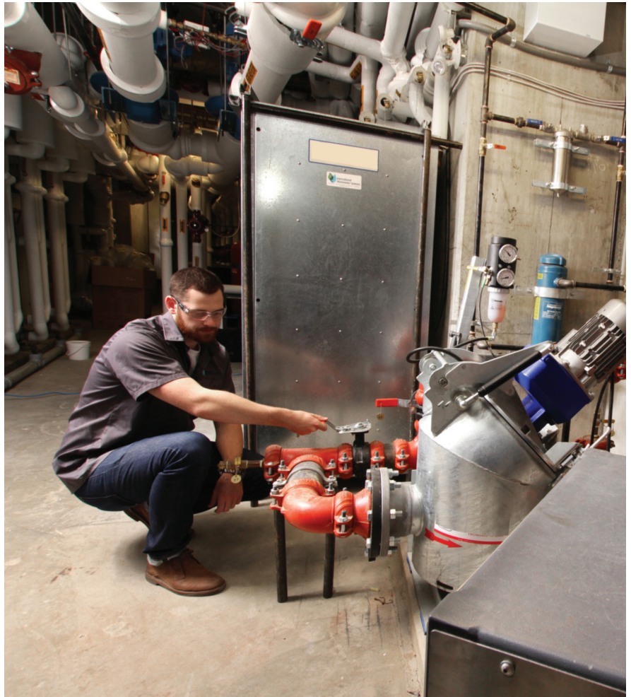
Raw sewage enters the system in the background and exits a filter in the foreground.
