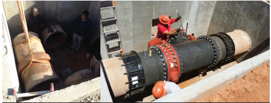
□ Workers replace part of the old piping. While repairs in the past required shutdowns, the new system of valves allowed work on parts of the system.
