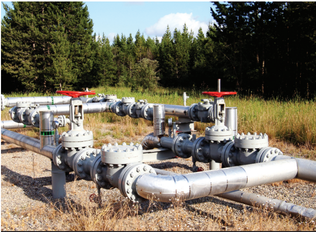
□ Many valves used in heavy oil transport lines are operated by hand.
