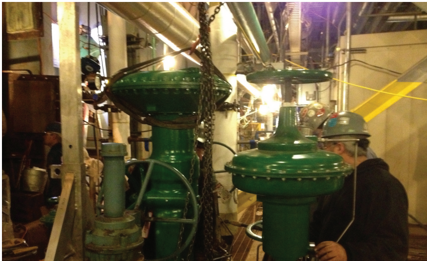
□ A control valve actuator is replaced in the lower elevation of BNYCP.
