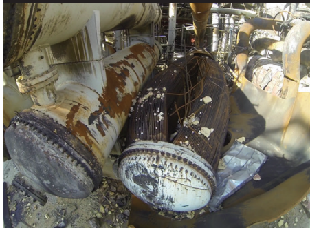
Figure 1. Post-blast photograph of the heat exchanger that ruptured catastrophically, causing extensive explosion and fire damage to the plant.
