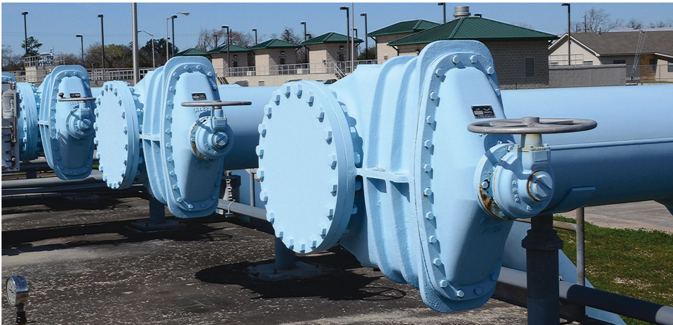
A trio of NPS 36, NRS gate valves are seen in manifolds at a water treatment facility.
