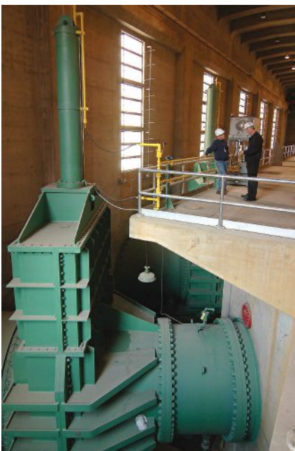
This is one of the eight 90-inch gate valves located in the bowels of Hoover Dam.
