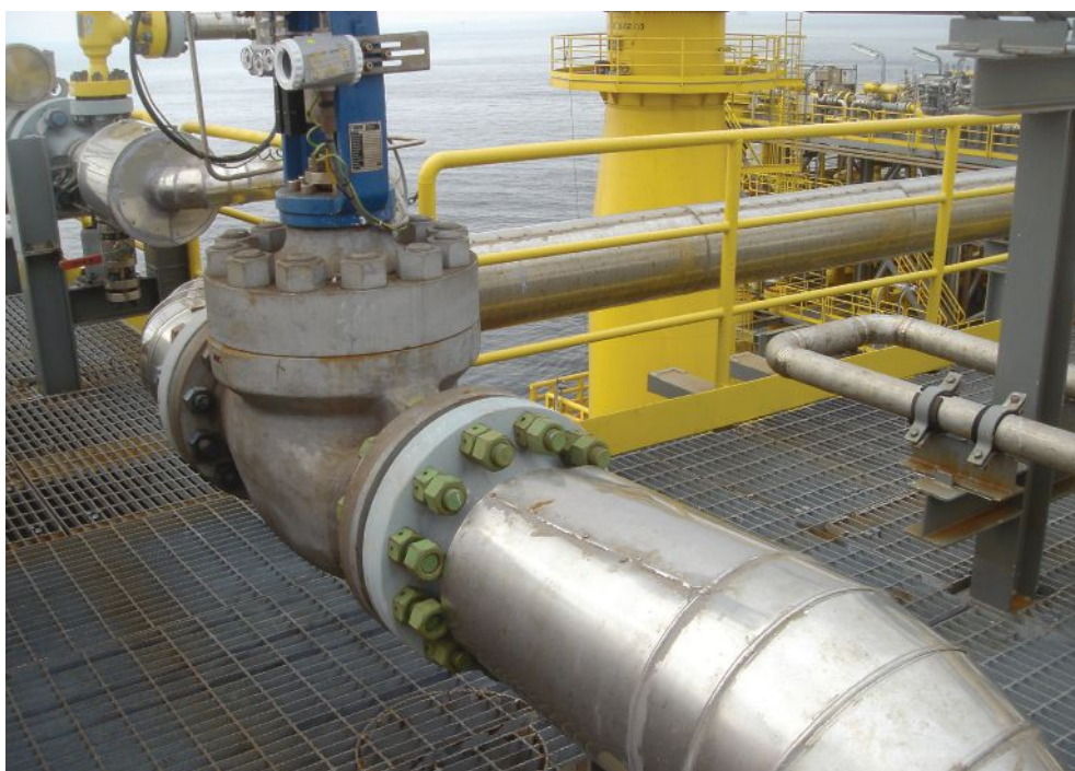
Typical valve offshore situated close to bends.
