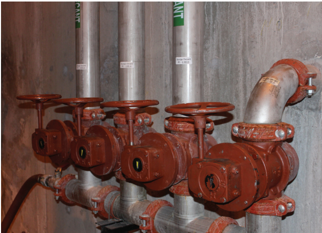
□ Some manually actuated valves are used in the system for purposes such as controlling raw sewage as it flows into areas where debris will be removed.
