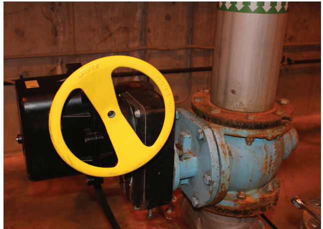
□ The plant works with local contractors to get special parts such as a repair kit for this obsolete plug valve.
