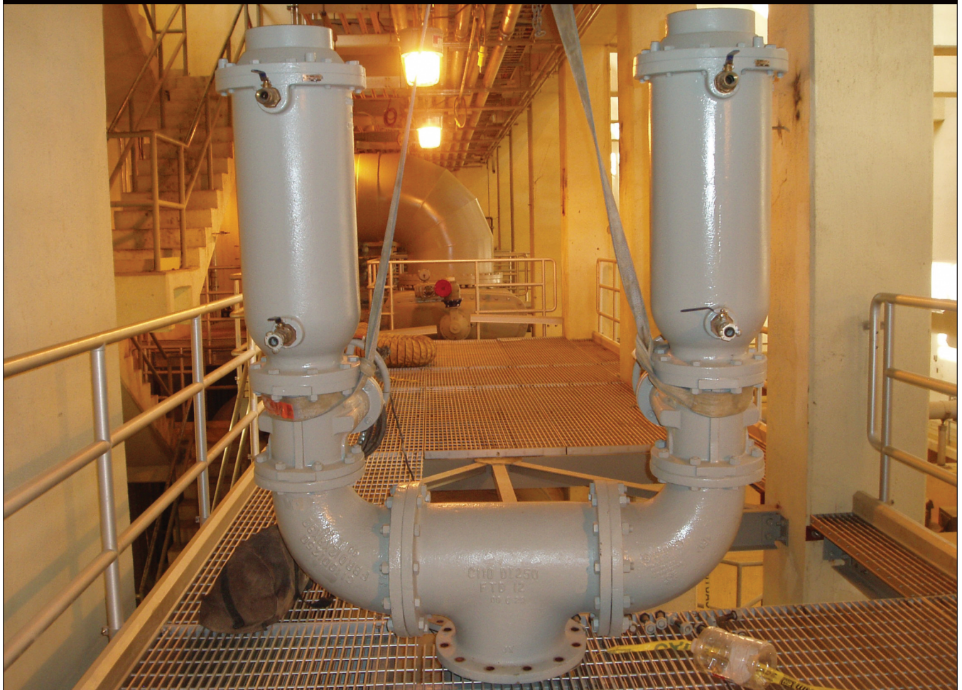
□ Wastewater air valves isolated by gate valves are installed in a wastewater treatment plant.
