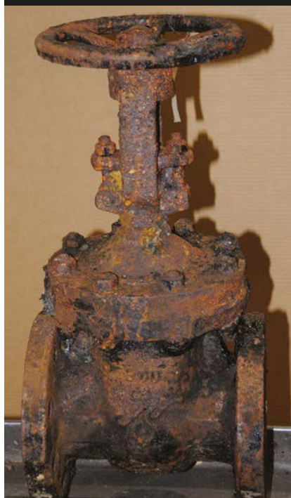
□ Sometimes it's more cost effective to replace a valve than to repair it, though if necessary, even this hulk could be refurbished and returned to service.
