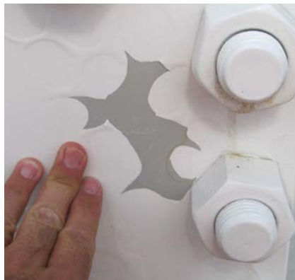
□ Figure 3. Blisters and topcoat delamination on a valve
