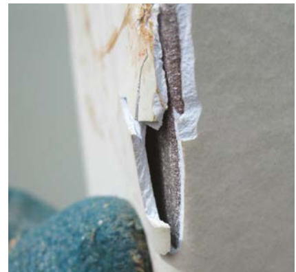
□ Figure 4. A small impact results in a much larger disbondment.
