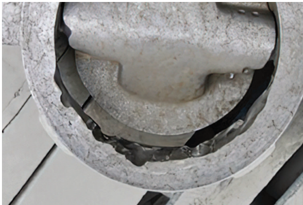
Metal seated butterfly valve damaged due to control of abrasive media. Source: SAF
