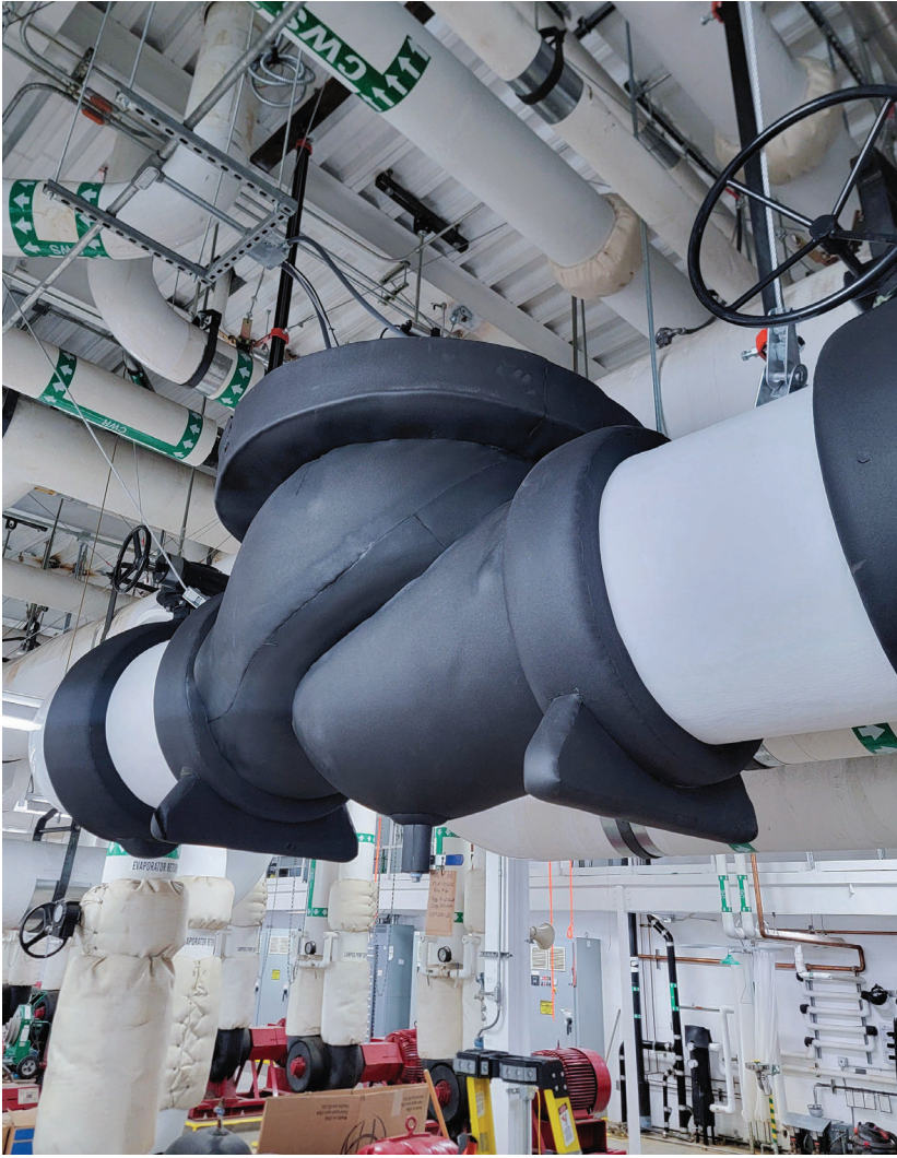
Valves encased in foam for a TES system.
