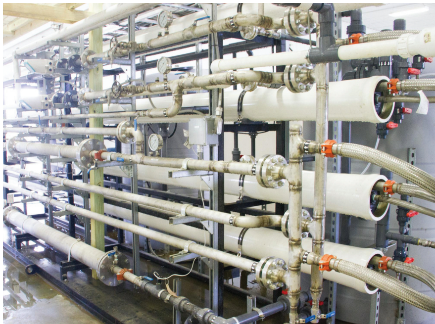
□ Pumps, piping and valves in the livestock recycling process
