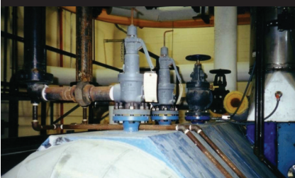
Figure 1. A fire-tube package boiler protected by two safety valves
