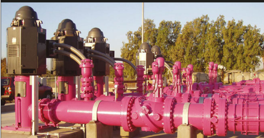
Figure 2. Air valves on pump discharge reduce air in pipelines in Chino, CA.
