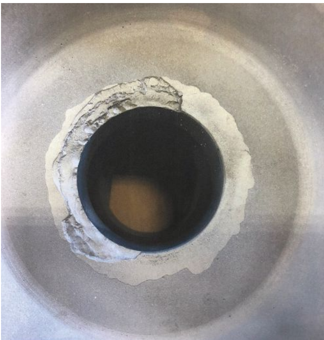
Cracked bonnet valve backseat before repairs were completed.
