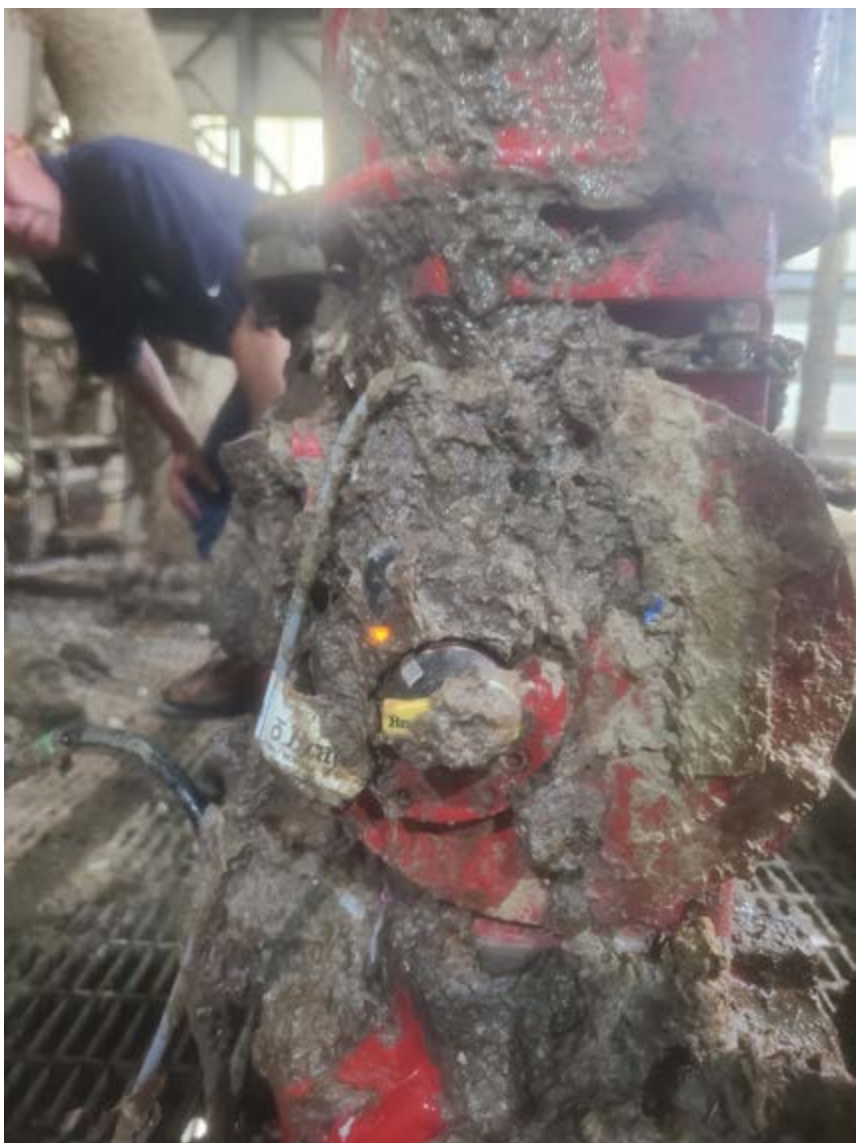
Actuator covered in pulp in application at a pulp recycling plant.
